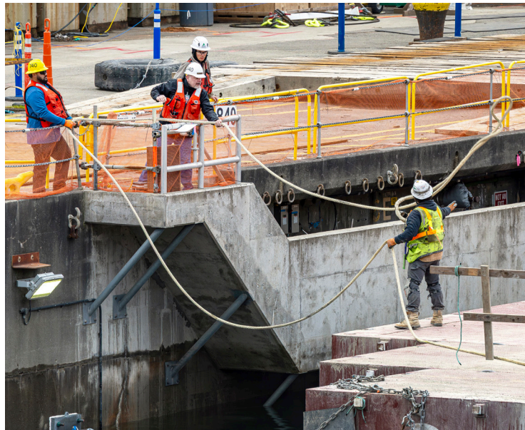
ABOVE: A team of Code 740, Riggers, works with Kiewit-Alberici contractors to move a barge loaded with equipment from Dry Dock 4, April 3, as the shipyard Seismic Retrofit Project completes its original scope of work. (U.S. Navy photo by Scott Hansen)
