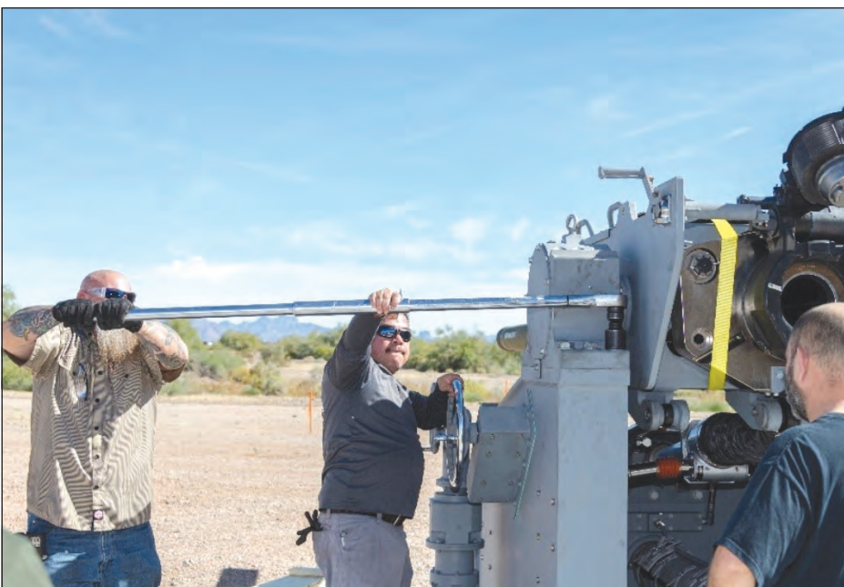
Crews used a special large pneumatic wrench to torque the mounting bolts to 3,100 foot-pounds. Then the carpenters constructed a wooden deck around the system to allow closer access to the Proof Gun System’s loading side.
