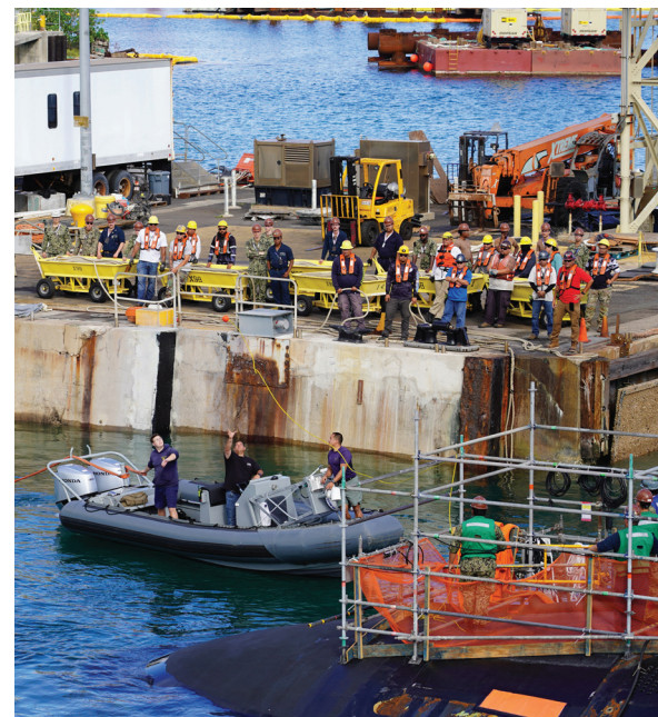
Code 760 Dive Locker personnel receive transfer lines during the recent docking of USS Colorado (SSN 788). The boat support provides a safety measure for in water issues and helps to safely pass lines from the dry dock walls to the vessel.
