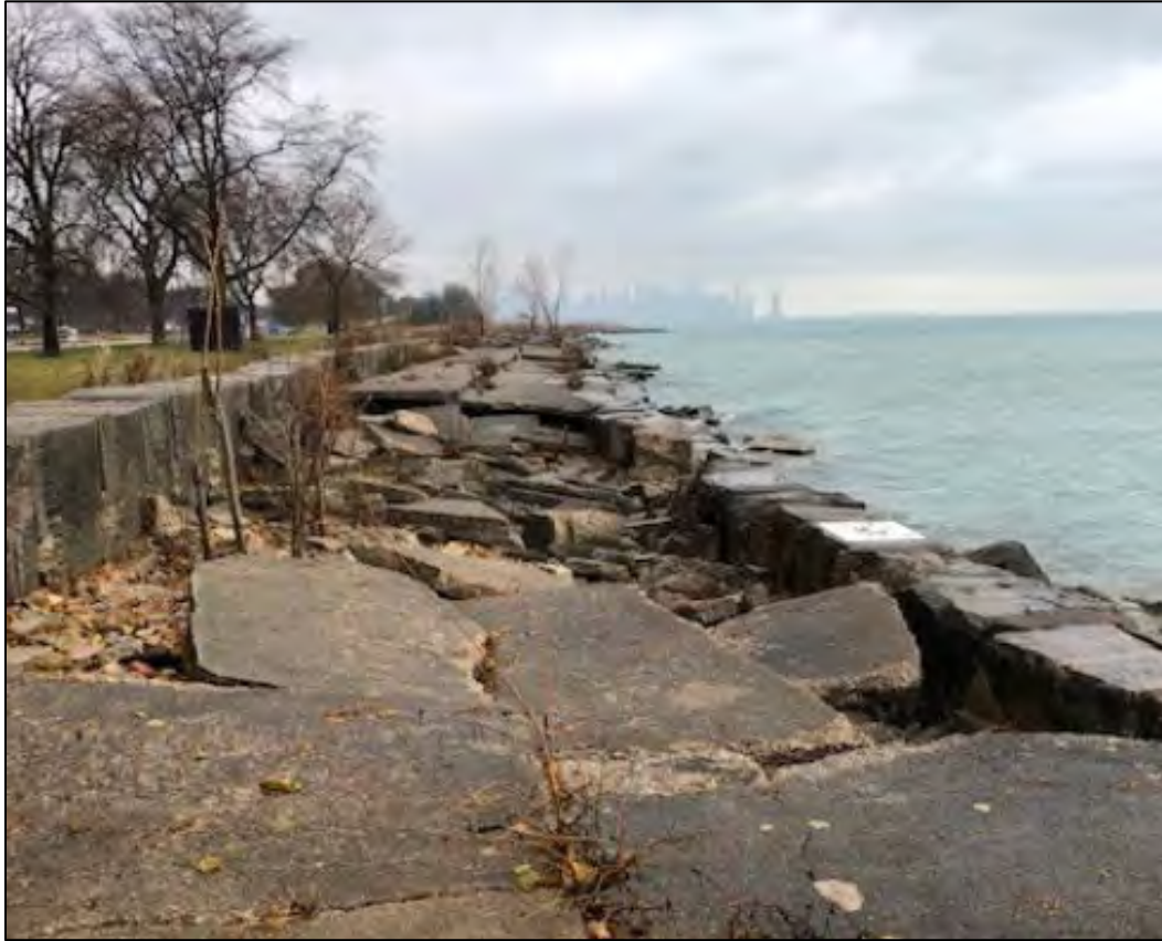
Figure 3: View of Existing Deteriorated Erosion Protection.
