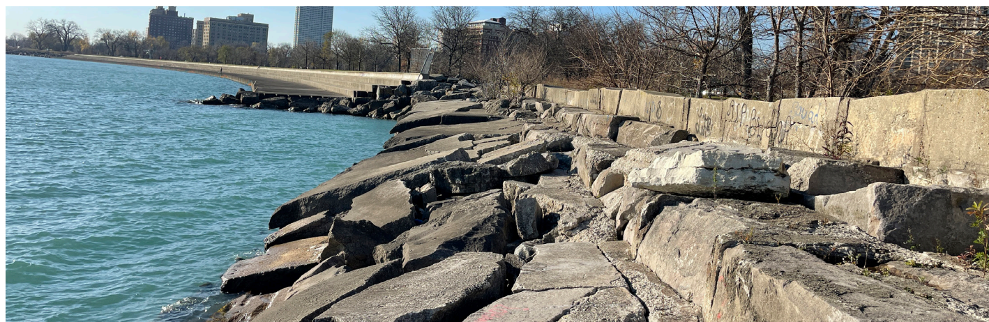
51st St existing concrete installed in 1970 is deteriorated and limits safe pedestrian access to water
