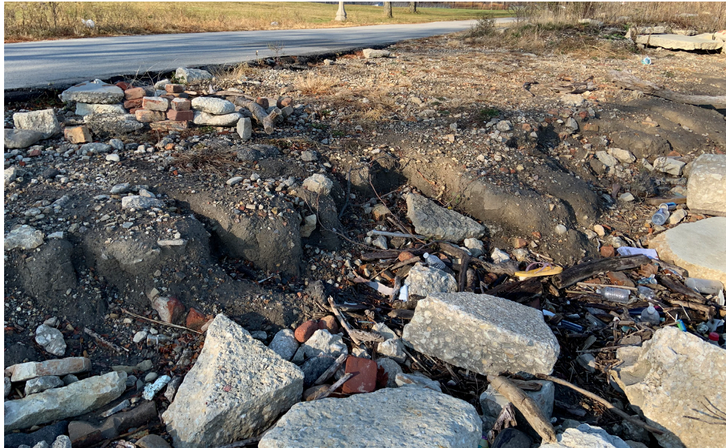
Active erosion and trail undermining prior to 2020 temporary measures.
