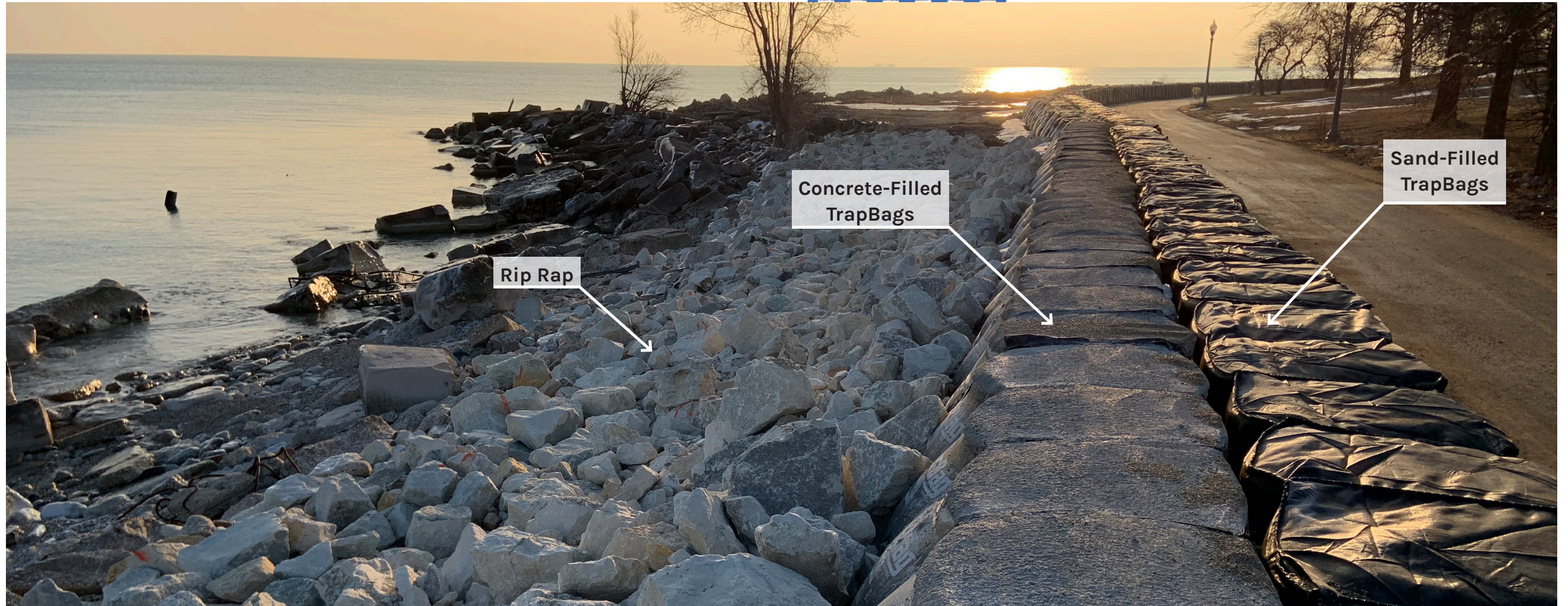
Deteriorating shoreline separated from pedestrian trail with temporary measures of rip rap and TrapBags.
