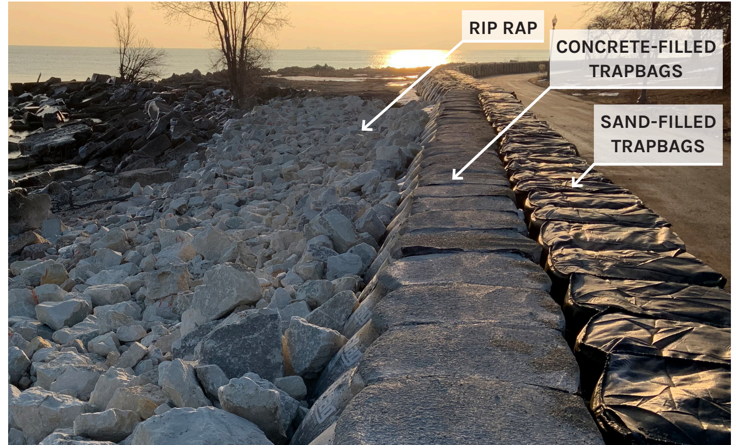
Deteriorating shoreline separated from pedestrian trail with temporary measures of rip rap and TrapBags.
