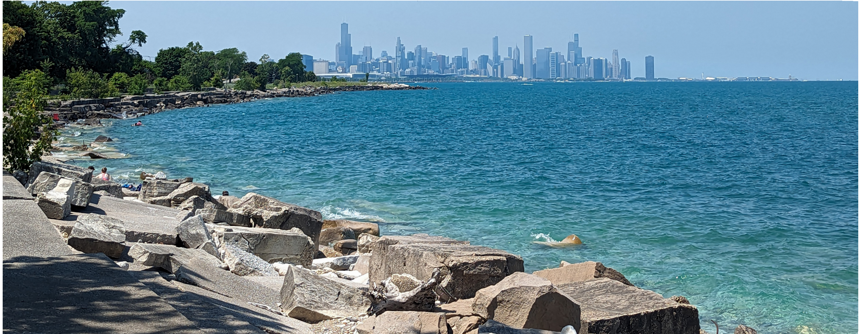
Existing edge of lakefront trail crumbling into the water limits areas where park visitors may safely interact with the lake.
