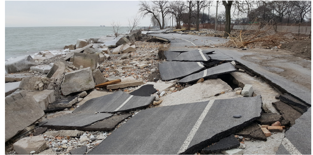
Destroyed lakefront path due to wave action
