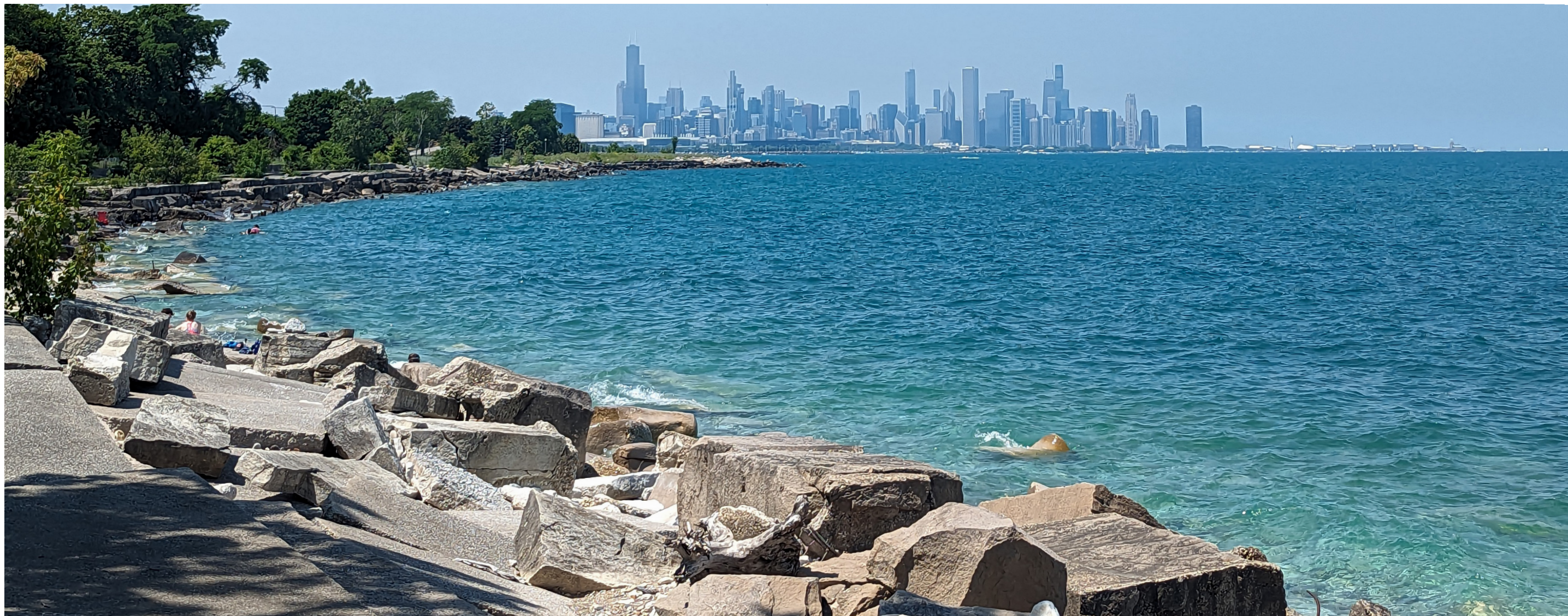
Existing edge of lakefront trail crumbling into the water limits areas where park visitors may safely interact with the lake.
