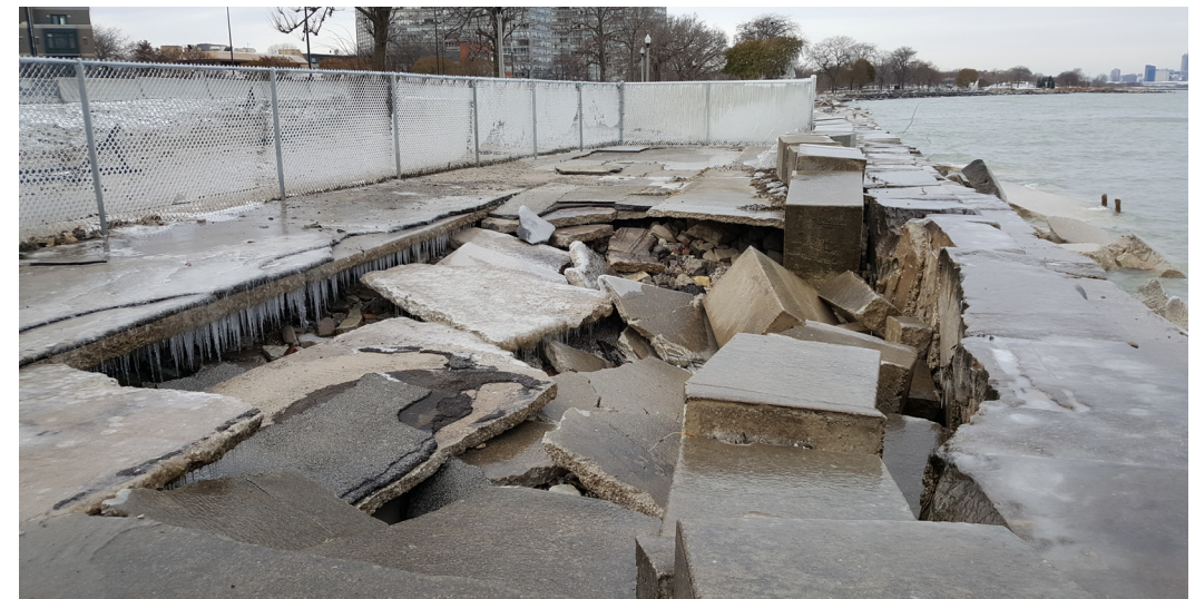
Collapsed concrete slabs and washout areas after winter storm
