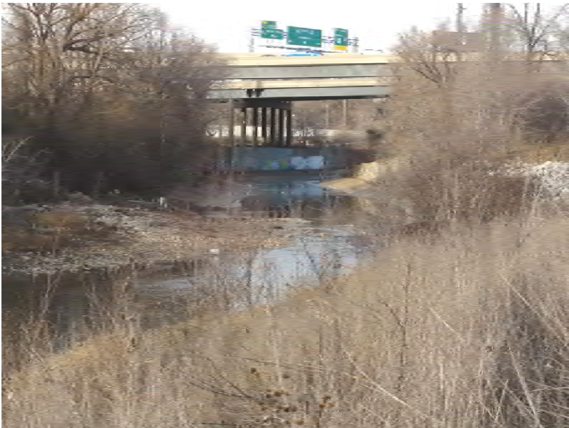
Figure 13: Menomonee River, downstream end of concrete lined channel showing sediment build-up
