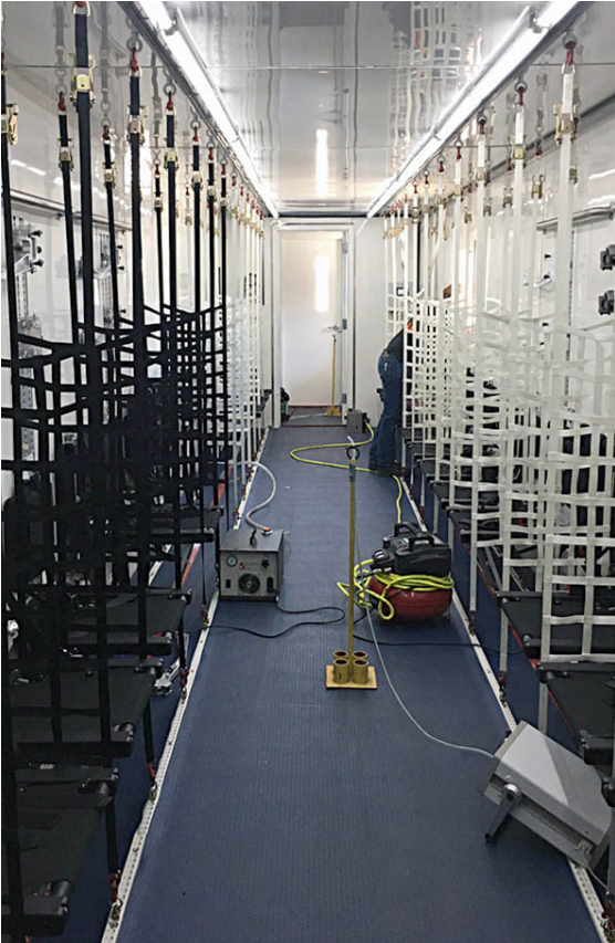
The interior of the negative pressure conex is pictured above. DCMA provided technical support and quality assurance to ensure the NPC met all specifications and requirement during its rapid development and fielding. (DCMA photo by Vern Lewis)
