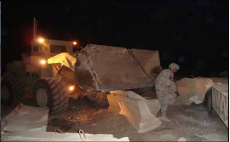
SGT Makii uses a loader and chains to yank jersey barriers from a trailer for disposal in the barrier yard.
