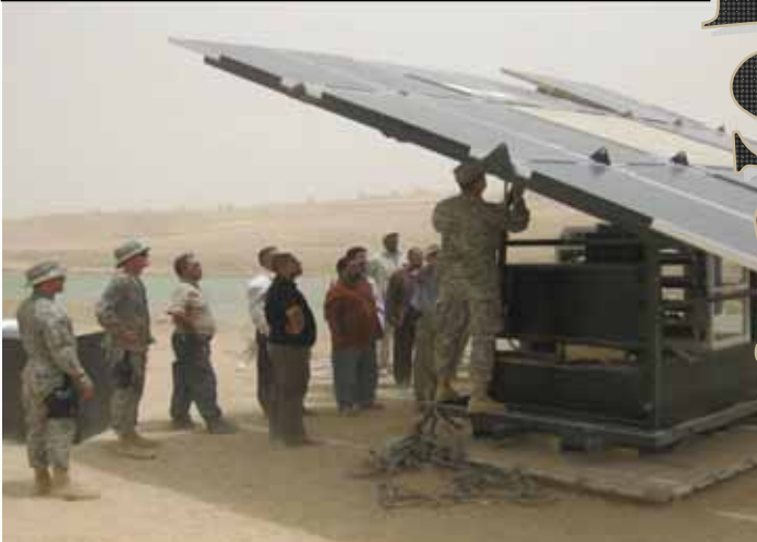
SSG Rogers (far right), demonstrates to Local National technicians the proper way to secure solar panels, while serving with Task Force Gold Forward.
