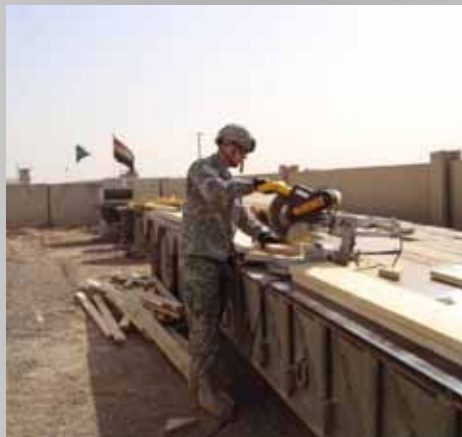
Spc. Robert Shoults, carpentry/masonry specialist from Berkeley, Mo., uses a miter saw while constructing the Joint Operations Center at Joint Security Station Shield.
