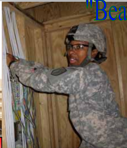
SGT Dixon preps an electrical panel box.
