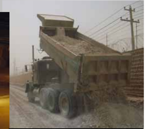
A heavy equipment operator drops gravel during road repairs on Camps Liberty/Victory.
