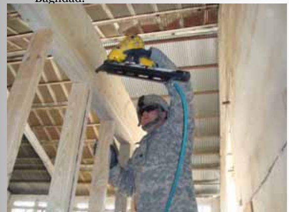
Right: Spc. Dale Webb, carpentry/masonry specialist from Ashland, Ohio, uses a nail gun to secure a top plate on the Joint Operations Center at Joint Security Station Shield.
