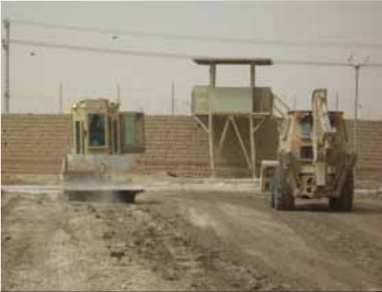
The smooth-faced roller compacts the roadway on Strawberry Hill Road in Baghdad.
