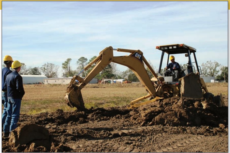
Louisiana National Guard Job Challenge Program cadet, 18-year-old Christian C. Morales of Puerto Rico, practices digging a trench using a backhoe in a remote field at the Gillis W. Long Center in Carville, La. JCP helps at-risk youth get back on track while receiving valuable job-skill training. Heavy equipment operator is one of eight trade certifications JCP has to offer. Photo: Staff Sgt. Stephanie J. Cross, State Aviation Command Unit
