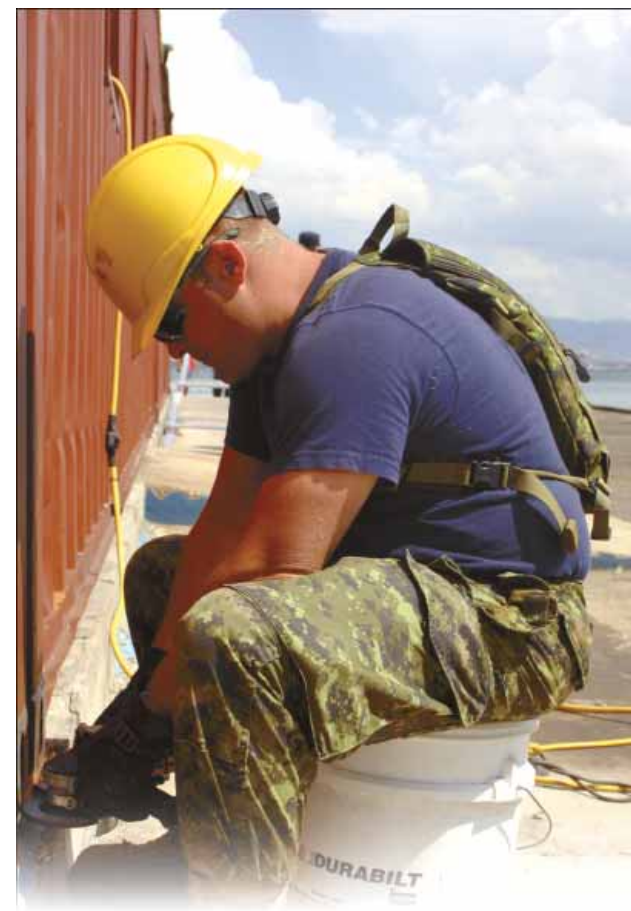
Cpl Dan Burkowsky, 192 AEF Aldergrove, grinds a sea container at Port Royal, one of the construction sites of EX TROPICAL HAMMER.
