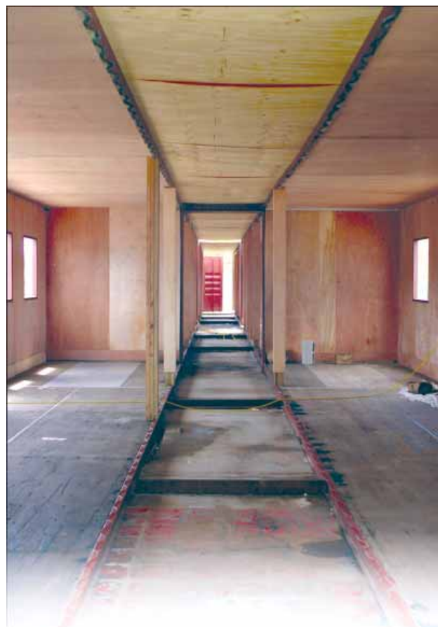
These soon to be accommodations being built at the Port Royal site are two sea containers welded together with space left in the centre for washrooms.
