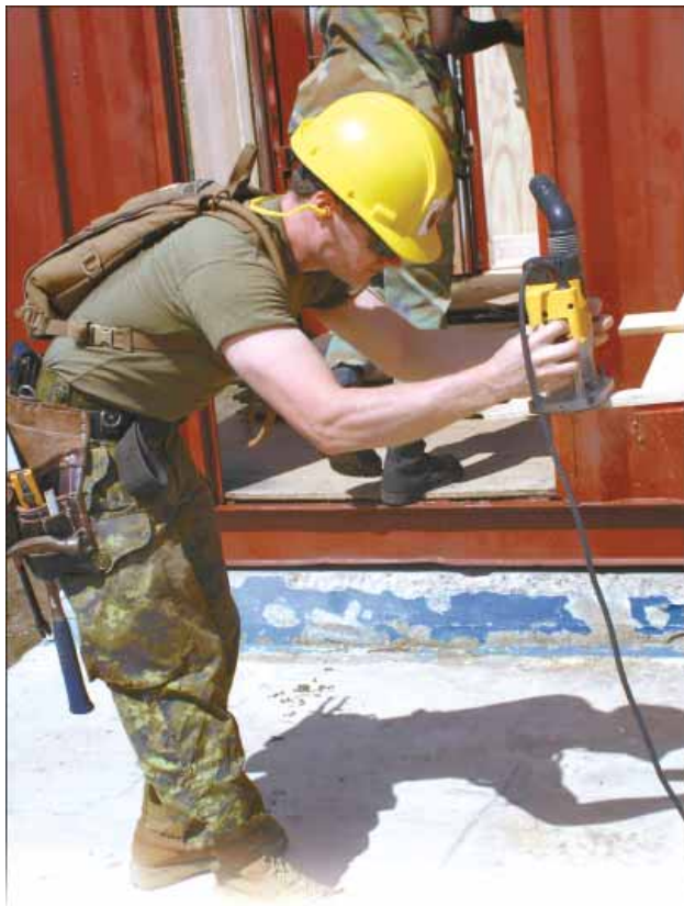
Cpl John Reith, of 191 AEF 19 Wing Comox, works a piece of plywood at the Port Royal site, part of Ex TROPICAL HAMMER.
