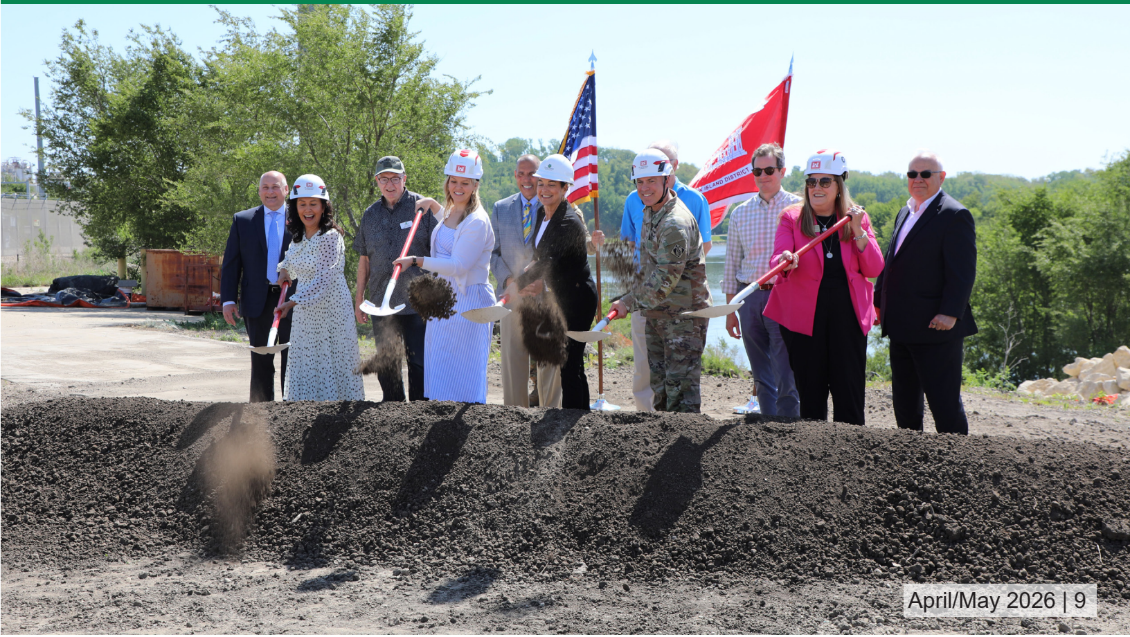
Below: With a flip of the shovel, the dirt is turned, and Reach 4, Phase 1 of the Cedar Rapids Flood Control System has officially begun. Photo by Frances Candelaria
