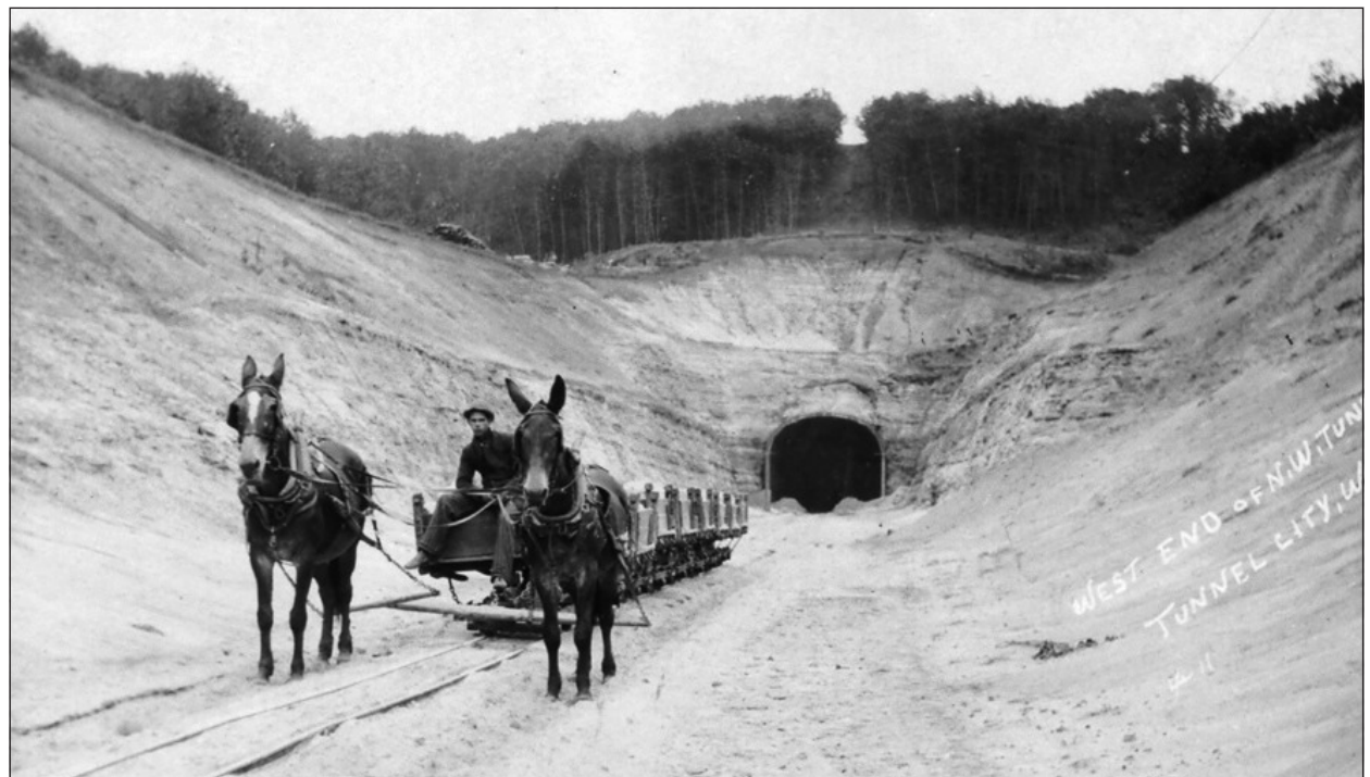
Photo shows construction work on the Chicago & North Western Railroad in Tunnel City, Wis., in 1911. Did you know that Monroe County has six railroad tunnels? Three are in Tunnel City and three are on what is now the Elroy-Sparta Bike Trail. This tunnel is located just a few miles from Fort McCoy.
