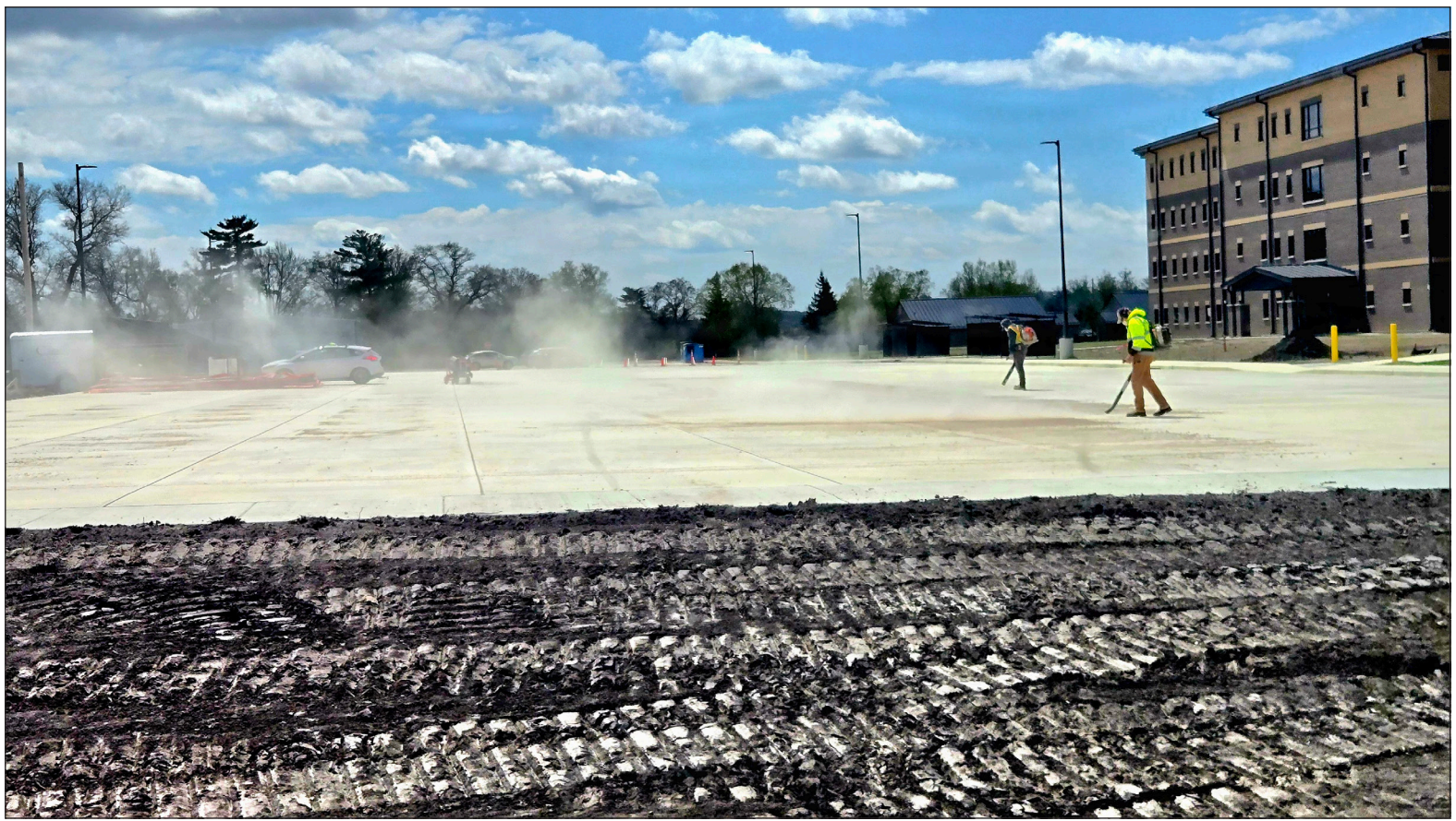
Contractors work on a new $27.3 million transient training troops barracks project, known as the Fort McCoy East Barracks Project, on May 7 at Fort McCoy.
