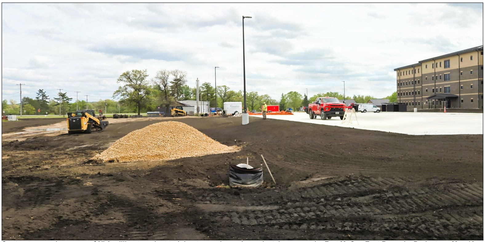
Contractors work on a new $27.3 million transient training troops barracks project, known as the Fort McCoy East Barracks Project, on May 18 at Fort McCoy.
