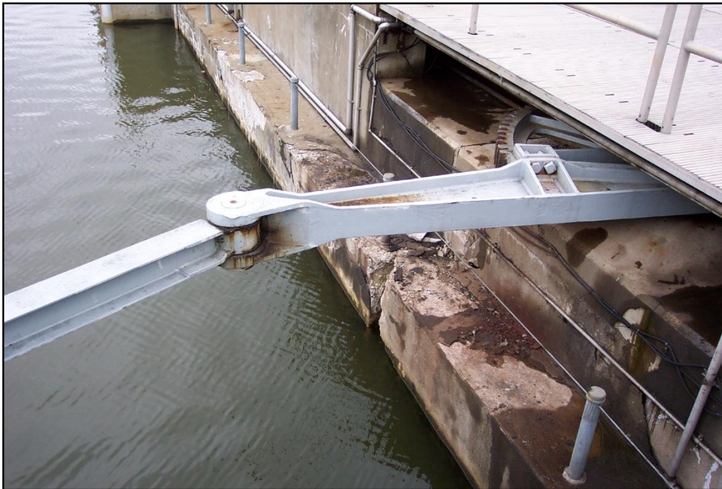
Photo 4-5: Miter Lock Gate Machinery (Arm)
