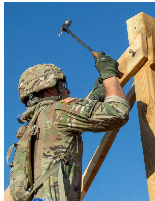
Top: Sgt. Mario Rancatore, a team leader assigned to 3rd Platoon, 859th Engineer Company, secures cross-bracing for a guard tower at McGregor Range Complex, New Mexico, July 25. (U.S. Army photo by Staff Sgt. Timothy Gray, 5th AR BDE)
