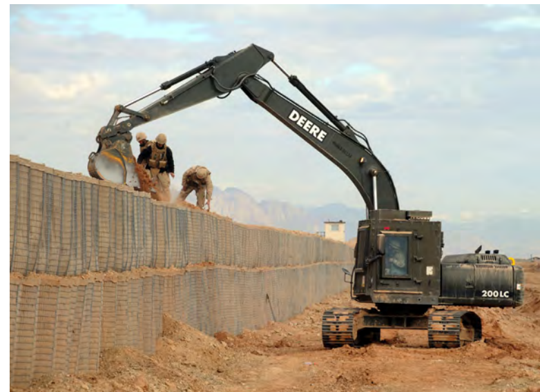
Seabees from Naval Mobile Construction Battalion 7 place dirt into Hesco protective barriers using an up-armored excavator at a forward operating base in Afghanistan on 25 January 2009. The unit was deployed to the country to provide construction support for contingency operations in support of NATO's International Security Assistance Forces.
