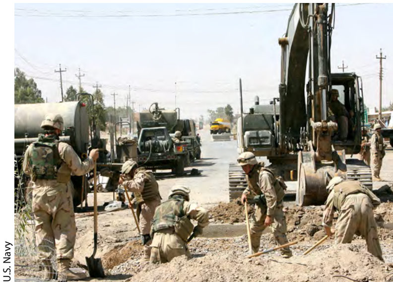
On 16 June 2006, Seabees began site preparation for construction of a bridge in Fallujah, Iraq. Personnel from Naval Mobile Construction Battalion 40 were tasked with rebuilding a damaged bridge that played a vital role for many Iraqi citizens. The battalion was deployed to provide essential support to coalition multi-national forces throughout Iraq.
