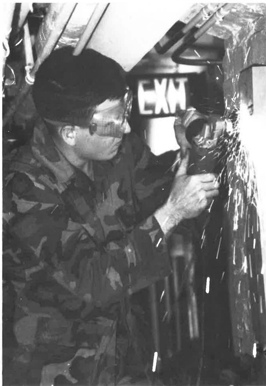
LCpl. Shawn Kelley, carpenter shop, works to install a door jam. This project took a little rigging to complete.
