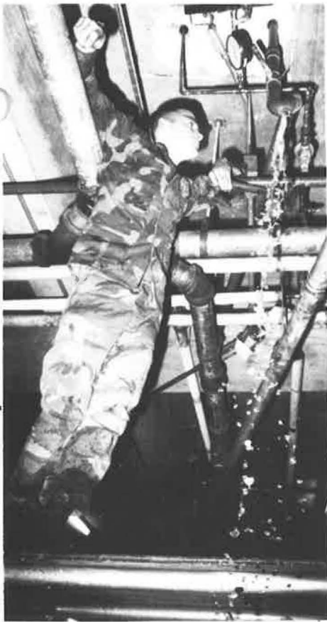
SSgt. "Buzz" Watts, snakes out some of the pipes in the UPL.
