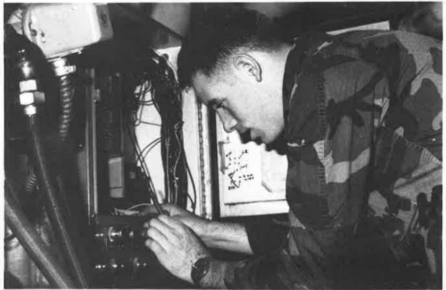
Cpl. Aaron Vincelette, boiler tech, makes sure the boiler is up to snuff.
