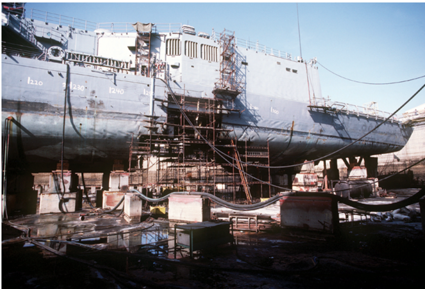
Samuel B. Roberts in drydock in Dubai undergoing repairs, revealing the scale of damage to the ship, 1988. (NARA, 6443425)
