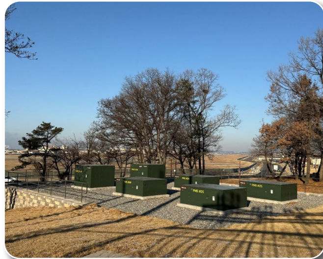
Power Supply Distribution System at Beacon Hill Switching Station, S-1451, Camp Humphreys
