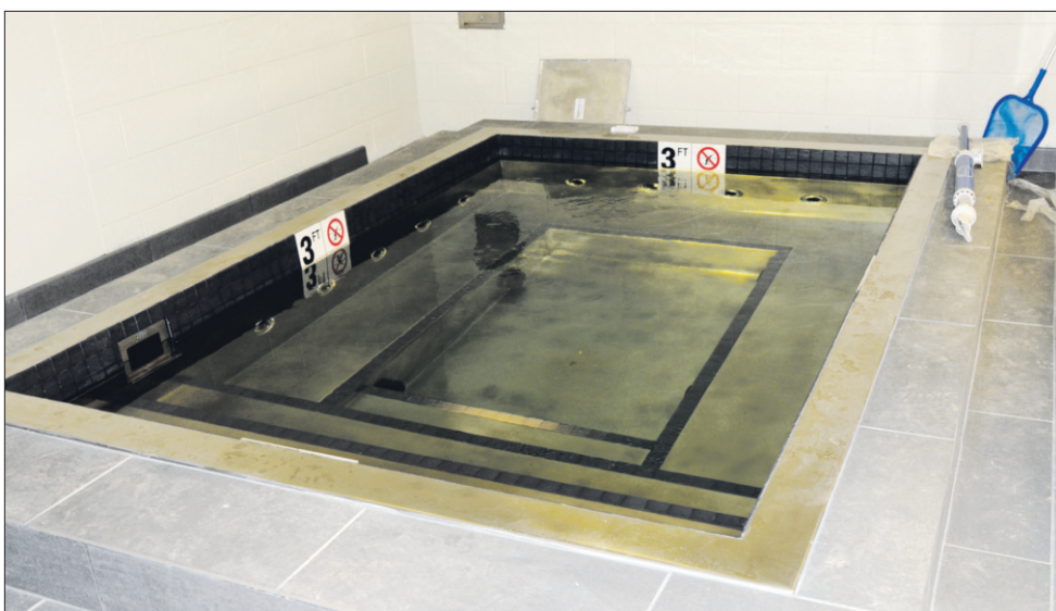
Whirlpools have been added to the latrines at the Camp Shelby Fitness Center Gymnasium.
