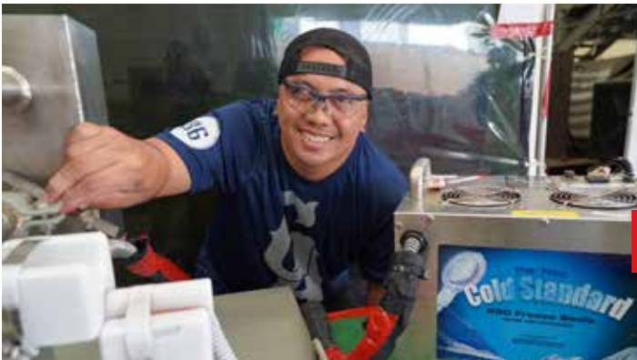
Shop 56 Pipefitter Mechanic Abraham Lobetos inspects Super Freeze equipment in support of USS Hawaii (SSN 776).
