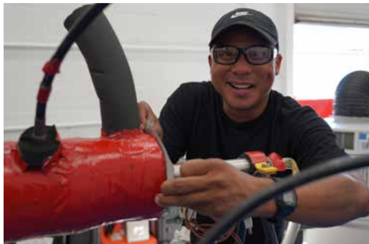
Shop 56 Nuclear Work Leader Benmar Pacubas installs the vortex freeze seal jacket. Freeze seals consist of an intentional mass of ice within a pipe that prevents water movement similar to a shut valve.
