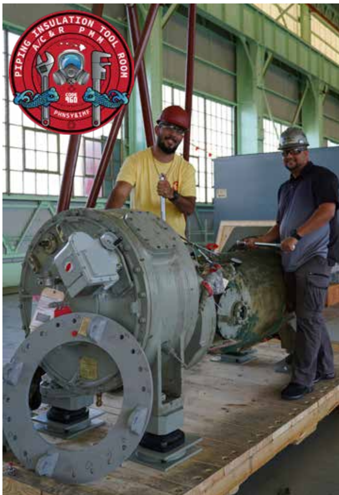
Shop Shop 56 ACR Work Leader Nainoa Sullivan and Shop 56 ACR Supervisor Johnathan Van Dyke are disassembling Air Conditioning components to ship to the OEM factory and Johnson Controls Inc. for analysis of the wear on internal components to determine future maintenance.
