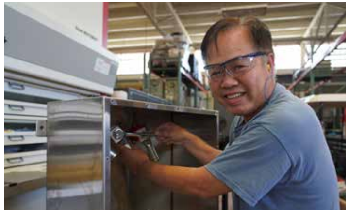
Shop 06 Electrician Mechanic Anthony Doan installs cam locks on a chill water electrical panel.
