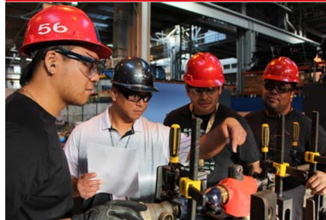
Code 960 General Foreman Todd Dumalao oversees Code 960 Apprentice Pipefitters Robert Ige and Ricky Duron and Code 960 Pipefitter Helper Roy Tamanaha with a pipefitting alignment that will support USS North Carolina (SSN-777.)
