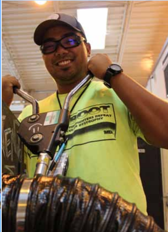
Code 990 first year Sheet Metal Apprentice Zachary Kaneshiro is finishing up the assembly of the ventilation tubing. The ventilation tubing can be as small as 4" to as big as 12" is used to supply positive air like the DH or AC and negative air such as hepa, dust collector or general ventilation, is used to help air out all confined spaces, tanks and containments for all shops and codes.
