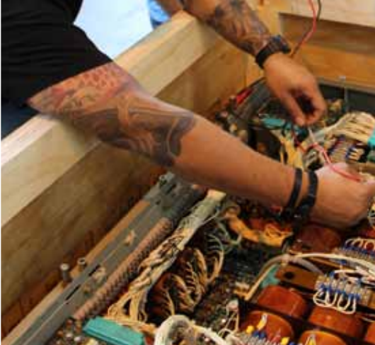
Code 950 first year Electrical Apprentices, Ryan Jacobs and Jacy Lau are in the Test Section performing resistance checks on an Insulated-Gate Bipolar Transistor (IGBT) voltage regulator.
