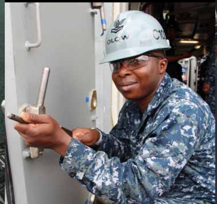
Code 103 Maintenance Assist team LeadMM1(SW) Abi Olowo, repairs Blast Doors onboard USS Port Royal (CG 73) prior to deployment.
