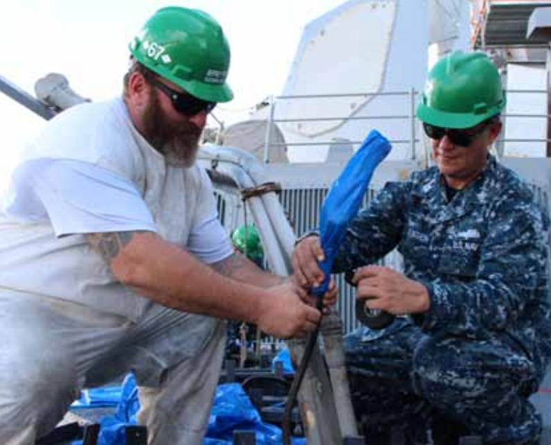
Code 950 Electrician GM1 Jensen assists Code 950 Electrical Work Leader Jeff Fortner weather proof cables on USS Halsey (DDG-97.)
