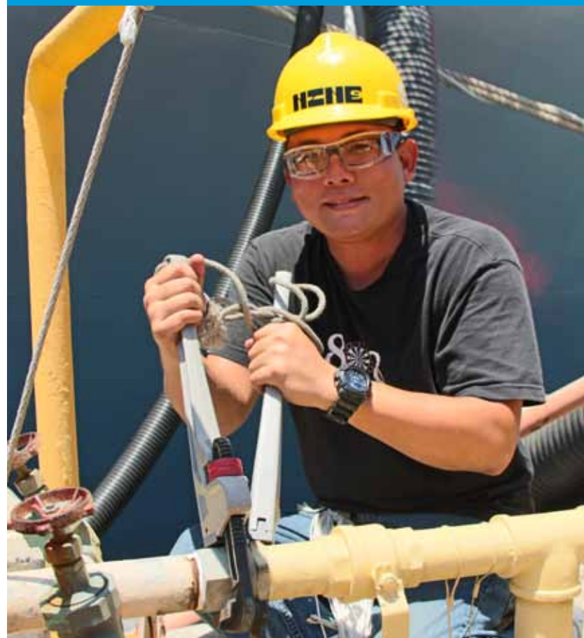
Code 990 Pipefitter Apprentice Dustin Maekawa tightens a riser to an air manifold. The air is distributed throughout the ship for pneumatic tools.
