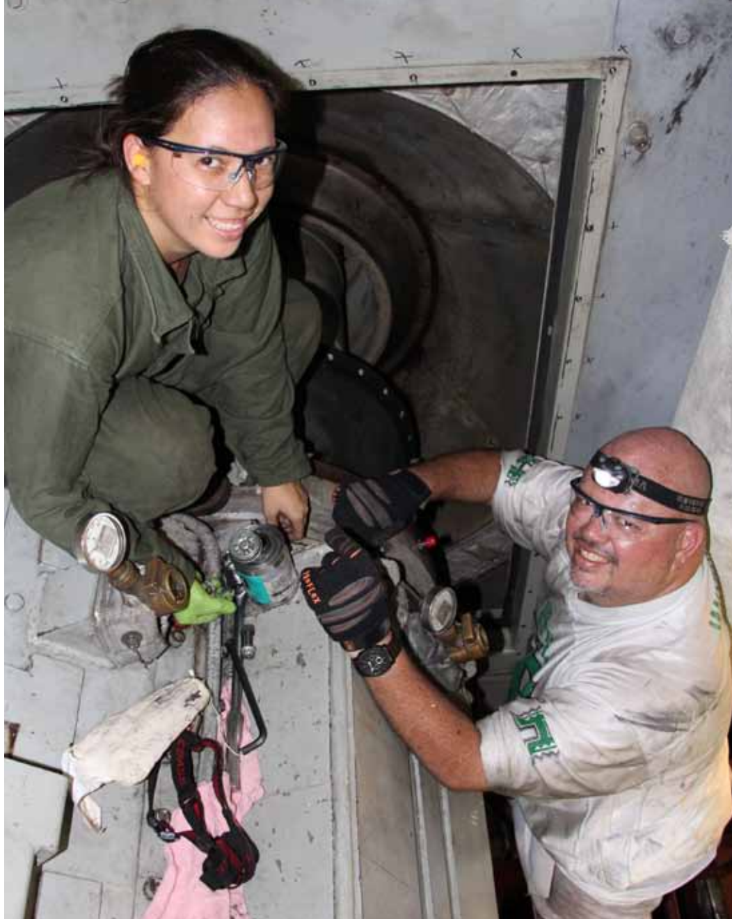
Code 930 Marine Machinist Work Leader Kanani Hawkins and Code 930 Marine Machinist Mechanic Nelson 'Alika' Barboza install a Power Turbine Brake on USS Hopper (DDG -70.)
