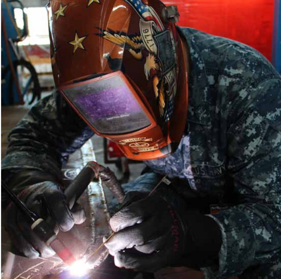
Code 920 Welder HT2 MacComber welds wedges and a new gasket channel to keep the doors water tight on USS Halsey (DDG-97.)
