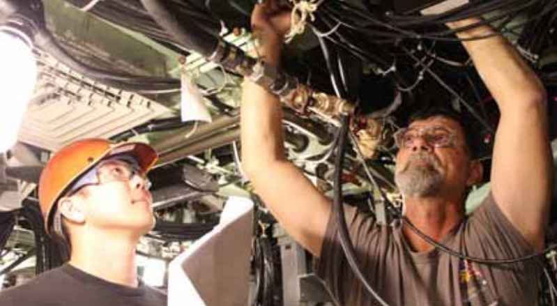
Electric Boat mechanic James Willis lays out the Fly-By Wire Ships Control System cable upgrade with Code 270 electrical engineer Radd Yatogo on USS Hawaii (SSN 776.)
