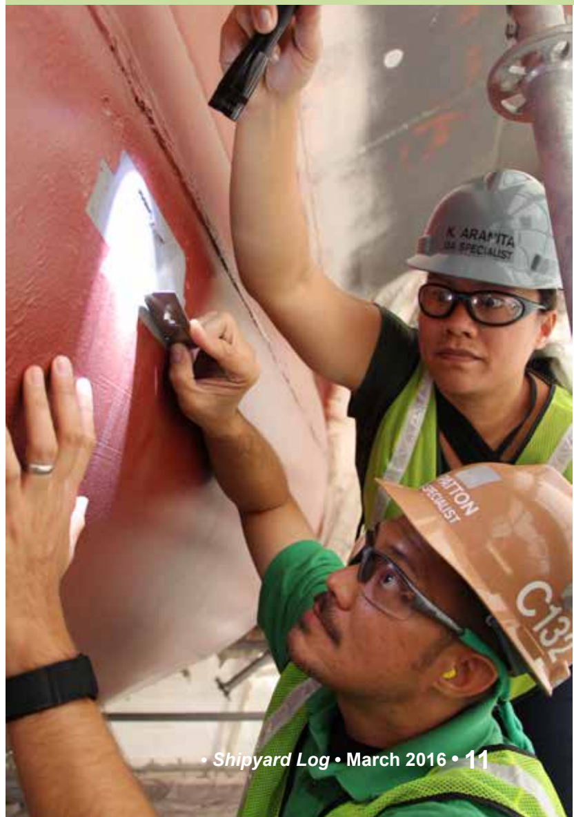
Code 132 Quality Assurance Specialists Lawrence Patton and Kauai Aranita provide government Nondestructive Testing oversight of contractor work on the external stern tube of a surface ship.
