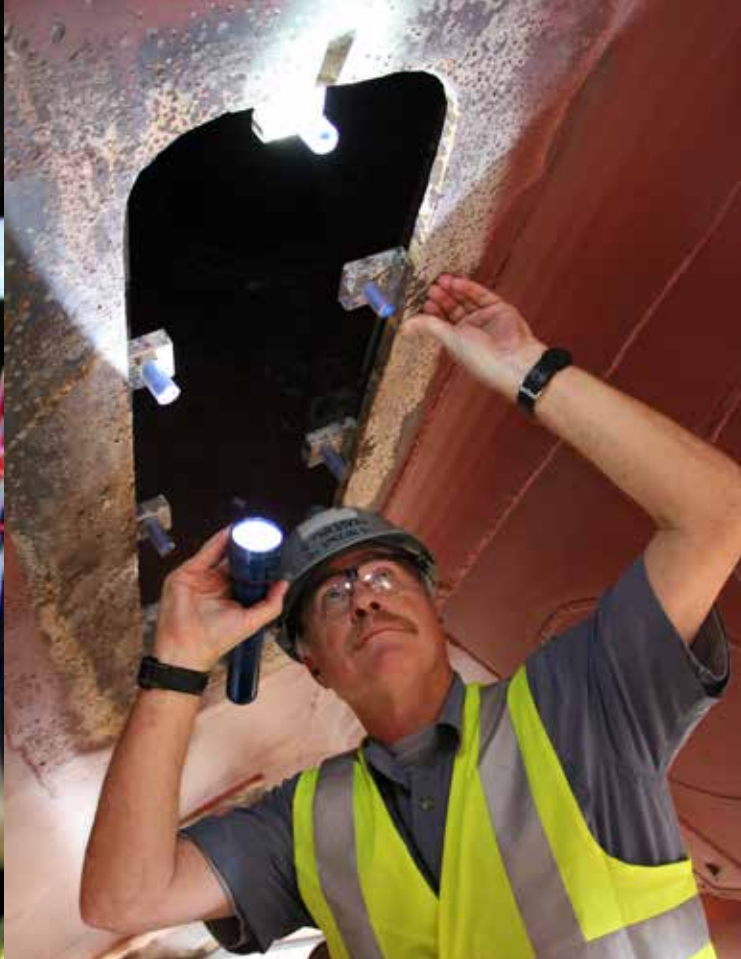
Code 132 Quality Assurance Inspector Gene Christmas conducts a critical surface ship coating inspection prior to blasting.
