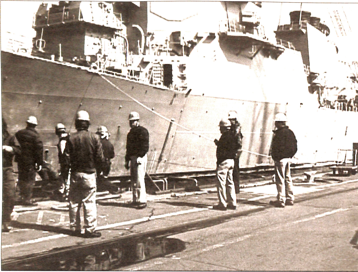
PERFECT FIT - Ship Repair Facility and Japan Regional Maintenance Center's cross-cultural workers bring USS Fitzgerald (DDG 62) into dry dock 5 for her emergency repairs.
