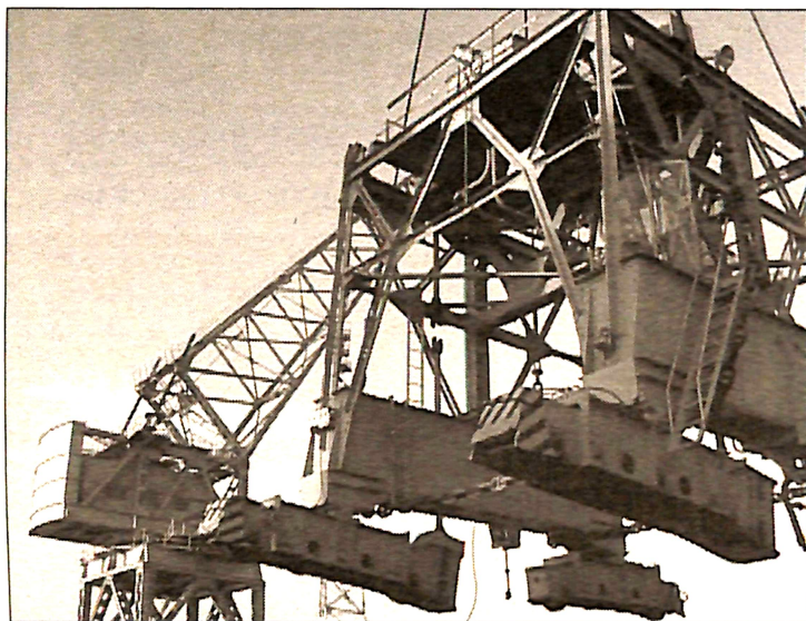
Workers from SRF, OICC and components demolish and remove one of the over 70-year old hammer-head cranes (LC-26) at SRF's Drydock No. 4.
