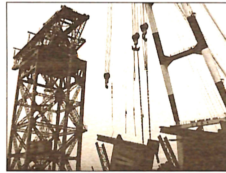
The Ship Repair Facility's 94-year-old land crane (LC 30) being dismantled at Berth 8. (Photo by Takahiro Takiguchi, CFAY Public Affairs)
