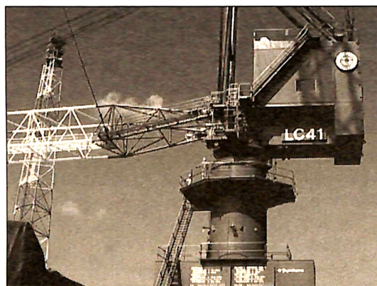
Ship Repair Facility installs a new 60-ton portal crane at Dry Dock No. 5.
