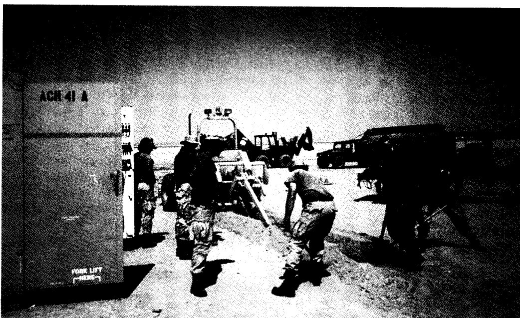
The hard-packed sand made it difficult to start construction. Here a team works on digging a trench.
