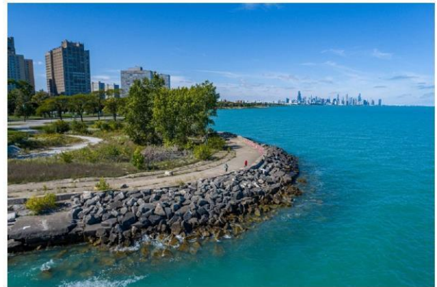
Figure 2-4. View of southern portion of project site near 51 st Street, looking north. The additional stone placed by the Chicago Park District several decades ago to protect an already damaged stepped revetment is clearly visible.
