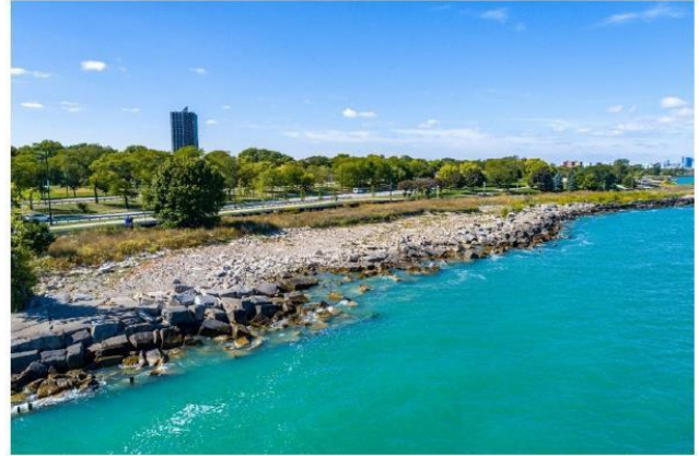
Figure 2-2. View of central portion of project site, looking north. Much of this area is no longer recognizable as having an engineered shore protection system. Nearly all of the capstones are displaced, and the area is undergoing active erosion.
