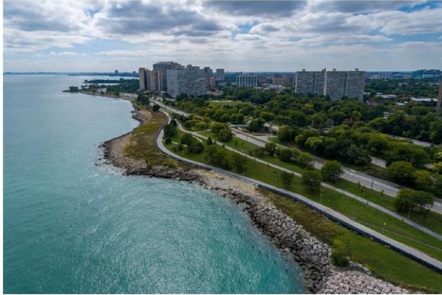
Figure 2-1. View of northern portion of project site, looking south. This area has been repeatedly repaired, and in 2020 emergency riprap and sand-filled TrapBags were placed to protect pedestrian trail from failure.
