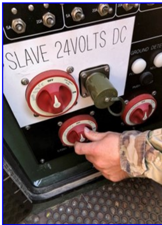
Turn OFF batteries on port (left) side of BEB.
