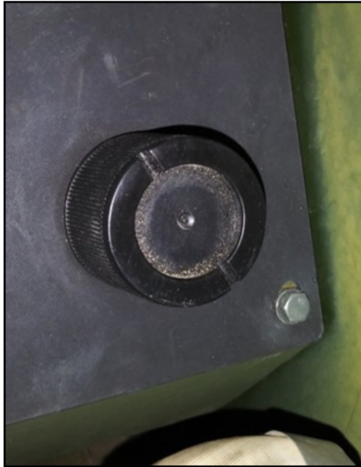
Lid placed atop air warning buzzer
