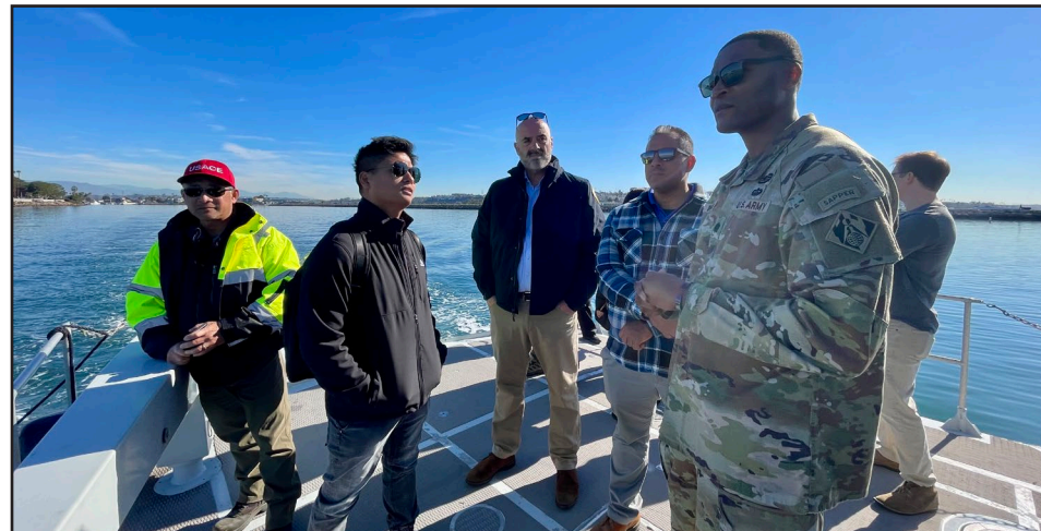
Lt. Col. Stephen Brooks, second from right, LA District deputy commander, joins project-delivery team members and LA County project partners on a Jan. 9 boat tour of dredging operations at Marina del Rey Harbor in LA County.
