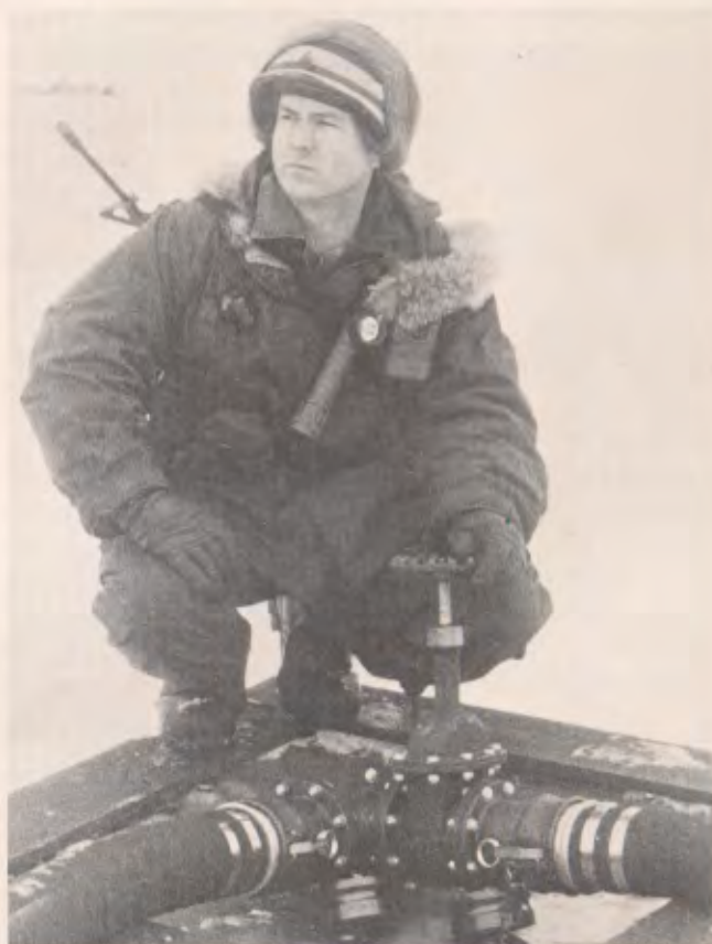
□ A soldier prepares to switch a valve during an emergency off-take point operation on the Central Europe Pipeline System.
