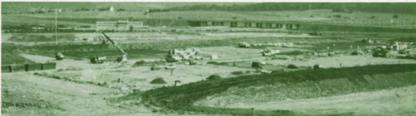
□ Bettembourg-Dudelange storage site is shown in the early days of construction, with major highway construction in the background.
