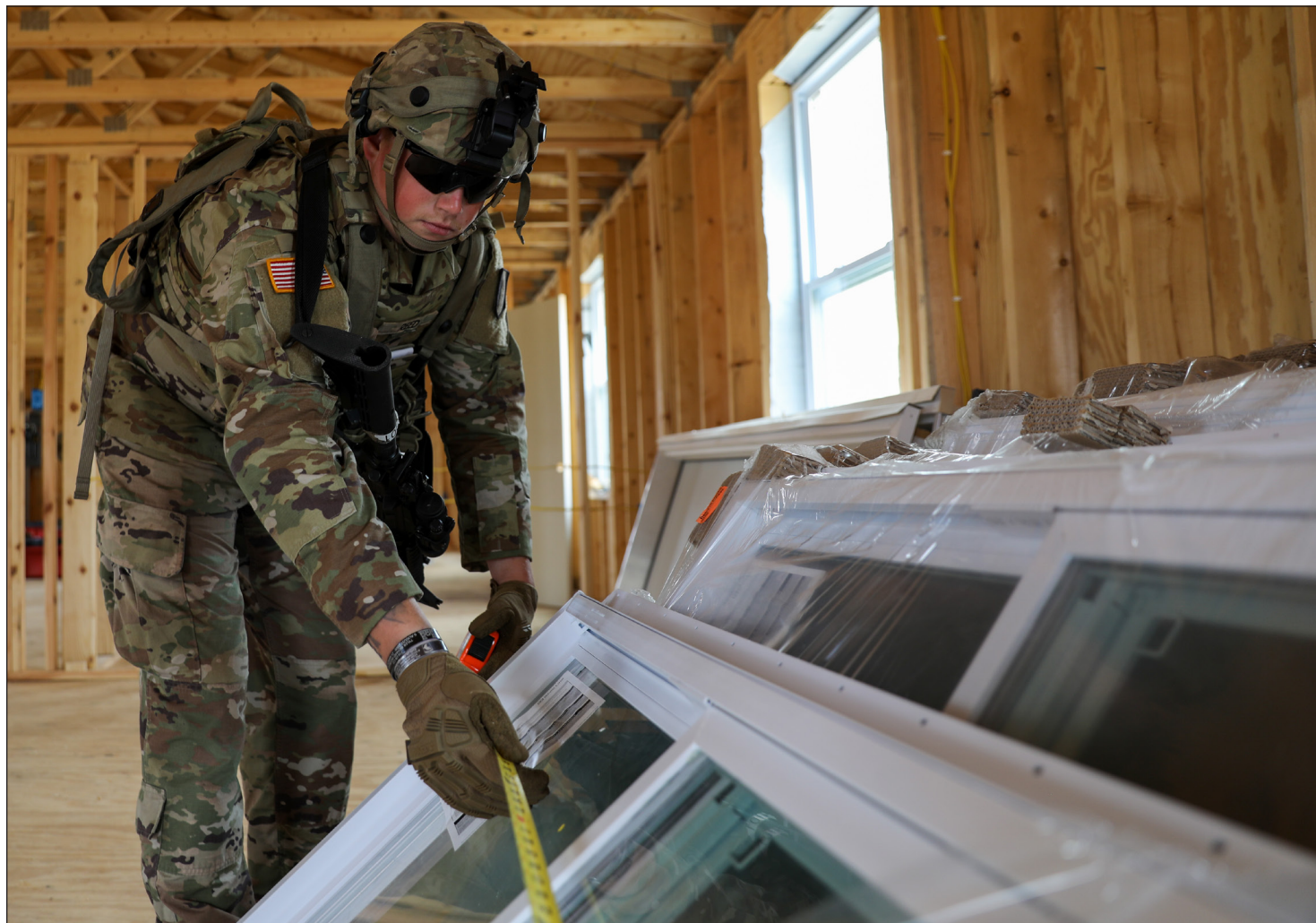
Spc. Christian Reed, a carpenter with the 716th Vertical Construction Company, measures a window Aug. 13 while working on a troop project to verify that the product meets building specifications during Combat Support Training Exercise 86-22-02 at Fort McCoy.
