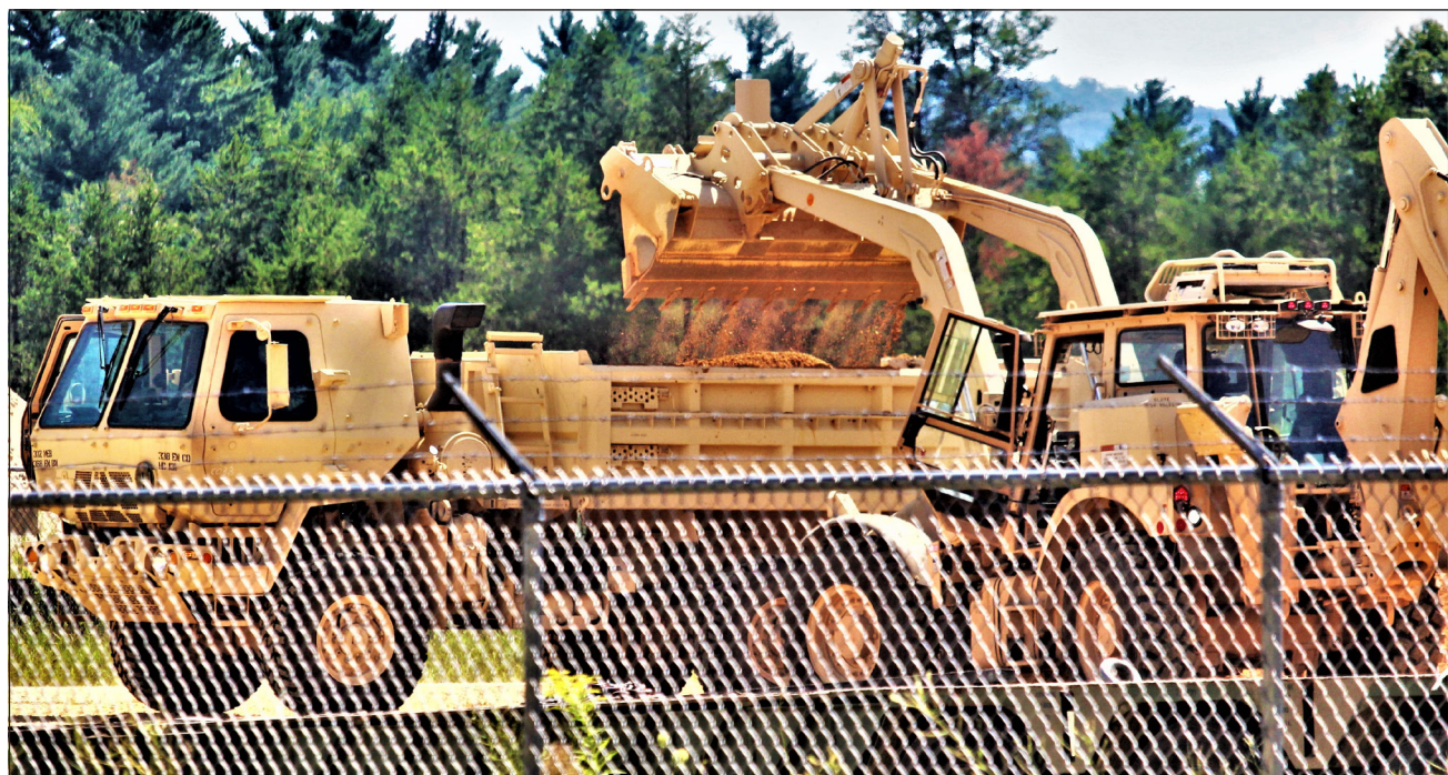
Soldiers with the 716th Engineer Company, an Army Reserve engineer company based in Summersville, N.H., work at the base operations support site troop project at Fort McCoy on Aug. 17 by moving fill dirt from the site.
