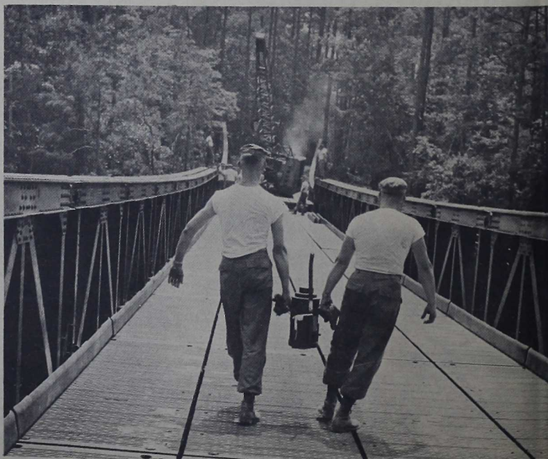
WORKING TOGETHER —Two men share the work carrying a hydraulic jack during construction of a M6 Fixed Panel Bridge. In the construction phases of training, the men learn how to work together for the completion of the mission.
