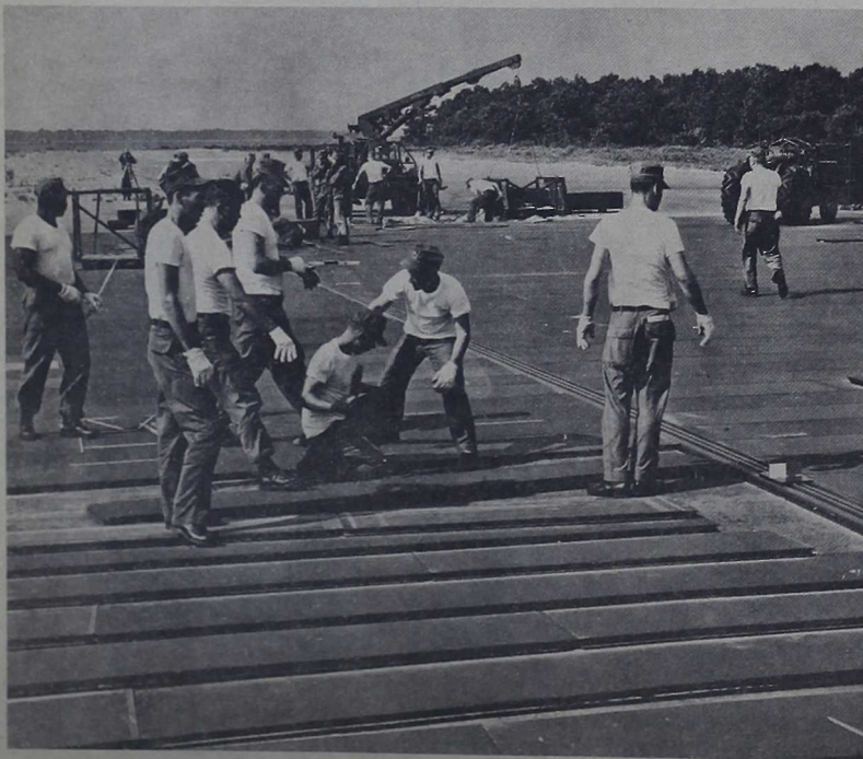
RUNWAY AND CATAPULT TRACK —Seabees lay the matting and the catapult track simultaneously during construction of the SATS runway at Bogue Field.
