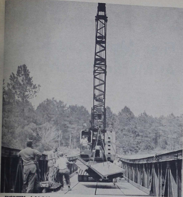
ENGINEERS of 2d Bridge Company, Force Troops, employ a crane to hoist the heavy metal section of deck panel into place during construction of a Fixed Panel Bridge. The use of a crane during construction can reduce man-hours by one-third.
