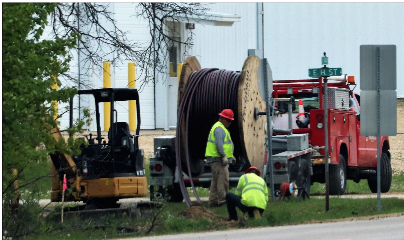
Contractors install underground power lines May 26 on the cantonment area at Fort McCoy. The work is part of an ongoing upgrade to Fort McCoy's electrical system.
