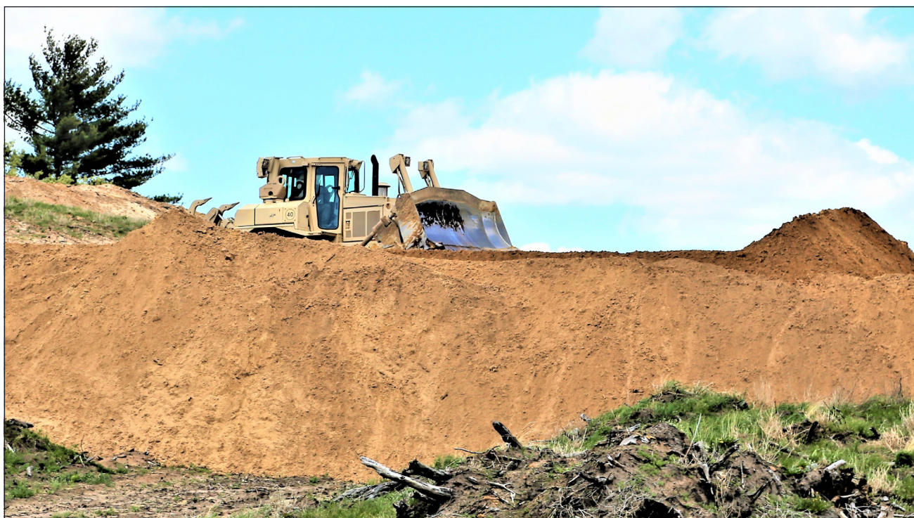
A Soldier with the Army Reserve's 372nd Engineer Company moves earth with a bulldozer May 16 as part of an ongoing troop construction project just outside the cantonment area fence at Fort McCoy. The project work is located in an area of land near the old Gate 20 and Improved Tactical Training Base Liberty and the cantonment area fence.
