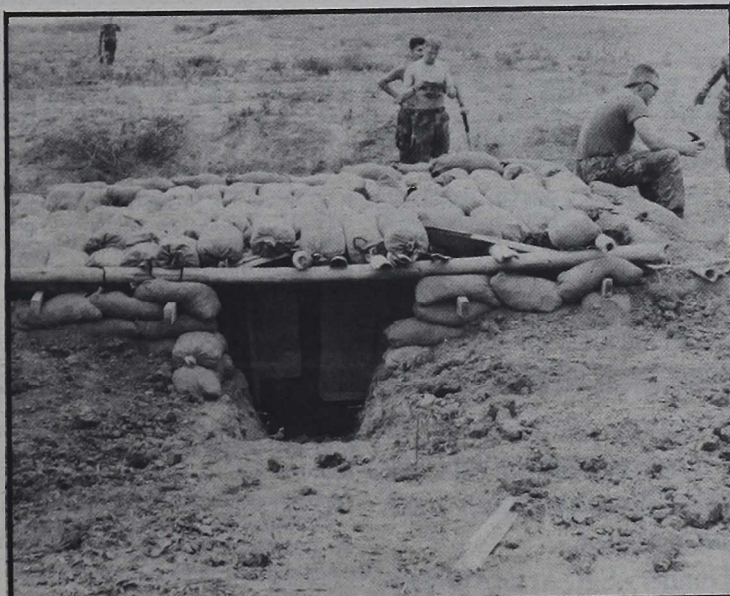
The field-expedient bunker constructed by U.S. Marines in UNITAS XXIX as seen from the rear entrance. Construction materials included empty mortar boxes, more than 200 sandbags and bamboo stalks found from the area.
