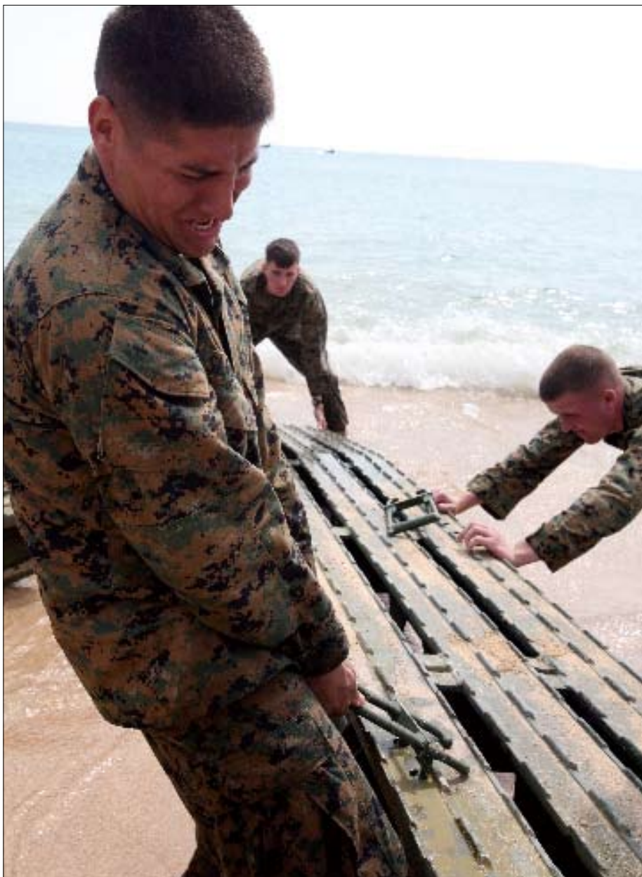
Pfc. Derek Slaughter, a combat engineer with 9th ESB, works to assemble a medium girder bridge at Kin Blue training area. Photo by Cpl. Monty Burton
