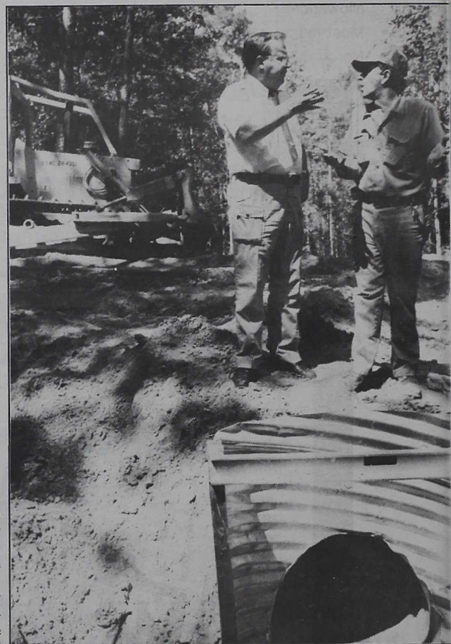
Charles Peterson, left, director, fish and wildlife division, MCB, discusses progress of green tree pond number three, with Don Goodson, a heavy equipment operator with Base Maintenance.
