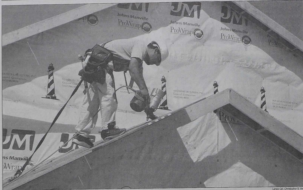
Workers with Harkins Builders Construction Company are placing the finishing touches on various base houses in the Midway Park housing district. Construction started in the middle of last year with the deconstruction of houses in the area.
