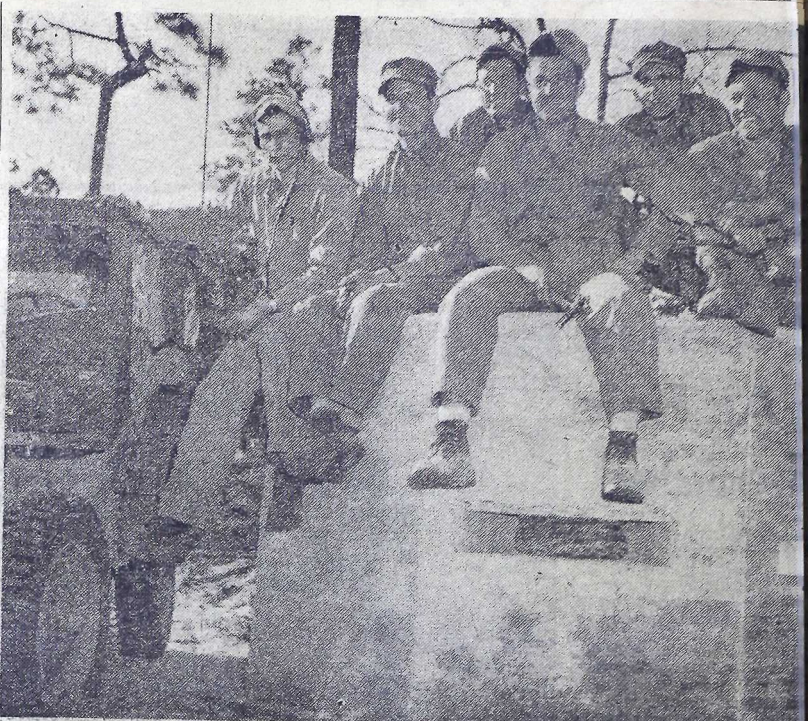
PILLBOX — Not long for this world is this brand new pillbox on which the engineers who "take ten." Located next to the 2d Tank Battalion Tank Park, the pillbox and nine others built, 2d Engineer Battalion are scheduled to be demolished in a demonstration of assault on a position Wednesday, March 7. Units of the Eighth Marines will do the "dirty work" before members of the North Carolina State Legislature invited here for the event by Gen. Ray A. Robinson. Members of the Headquarters Company Second Engineers, pictured above are, left to right: Cpl. A. F. DiMarzio, W. D. Hortman, Pfc. Jan Durand, Sgt. James M. Wolford, Sgt. Leonard A. Leonard, and Sgt. E. H. Nedy.
