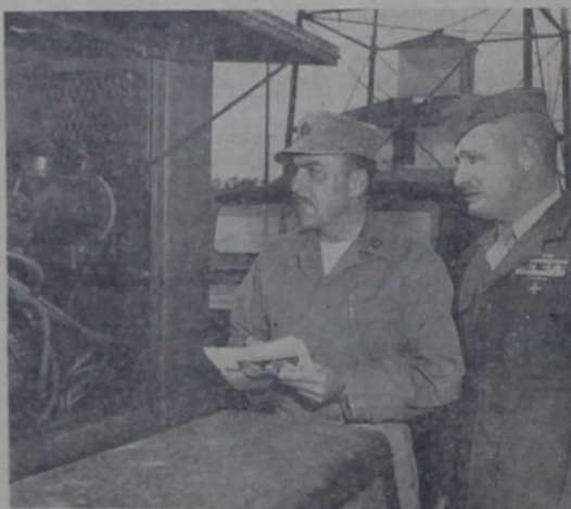
FIELD INSPECTION —Act. GySgt. Mike Rinaudo, left, and Comm 1st Sgt. Paul Oldaker check a trailer-generator. These portable electrical plants are called on for a variety of power-supply missions in the field.
