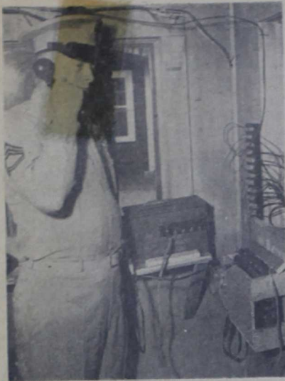
GYSGT. JAMES J. WALSH tests the original switchboard he helped design and build. This board was placed in the sentry booth at the entrance to the new ITR Supply Ammunition Point.
