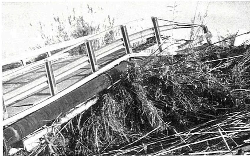
Giant reeds break loose from the stream bed and clog bridges.
