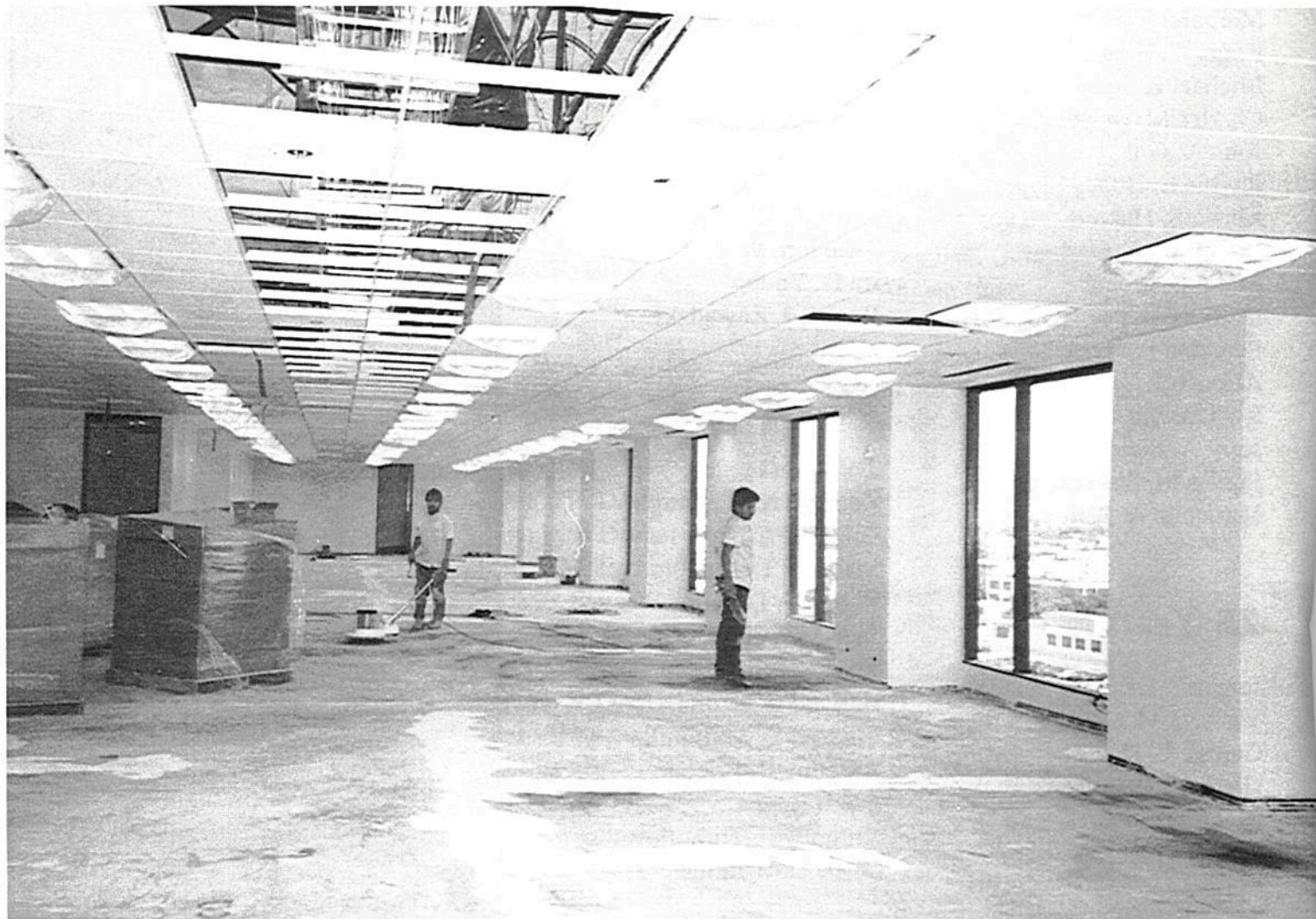
Before the District seriously started packing up, workmen were preparing the new building to receive nearly 600 Corps members.
