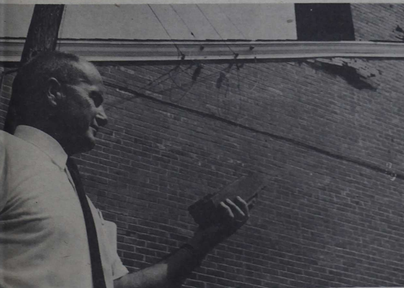
DEBRIS —Brewster Junior High School Assistant Principal, T.C. Webb holds one of the bricks knocked loose when a bolt of lightning struck a wall of the school.
